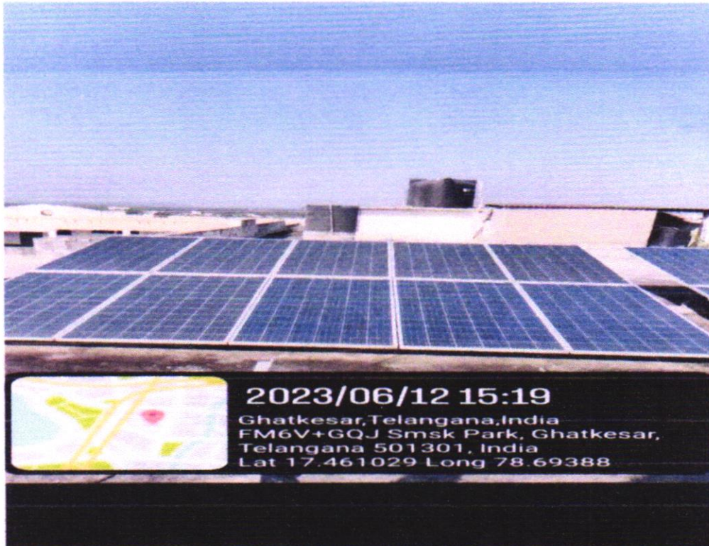
Image showing solar power panel installed on top of roof
